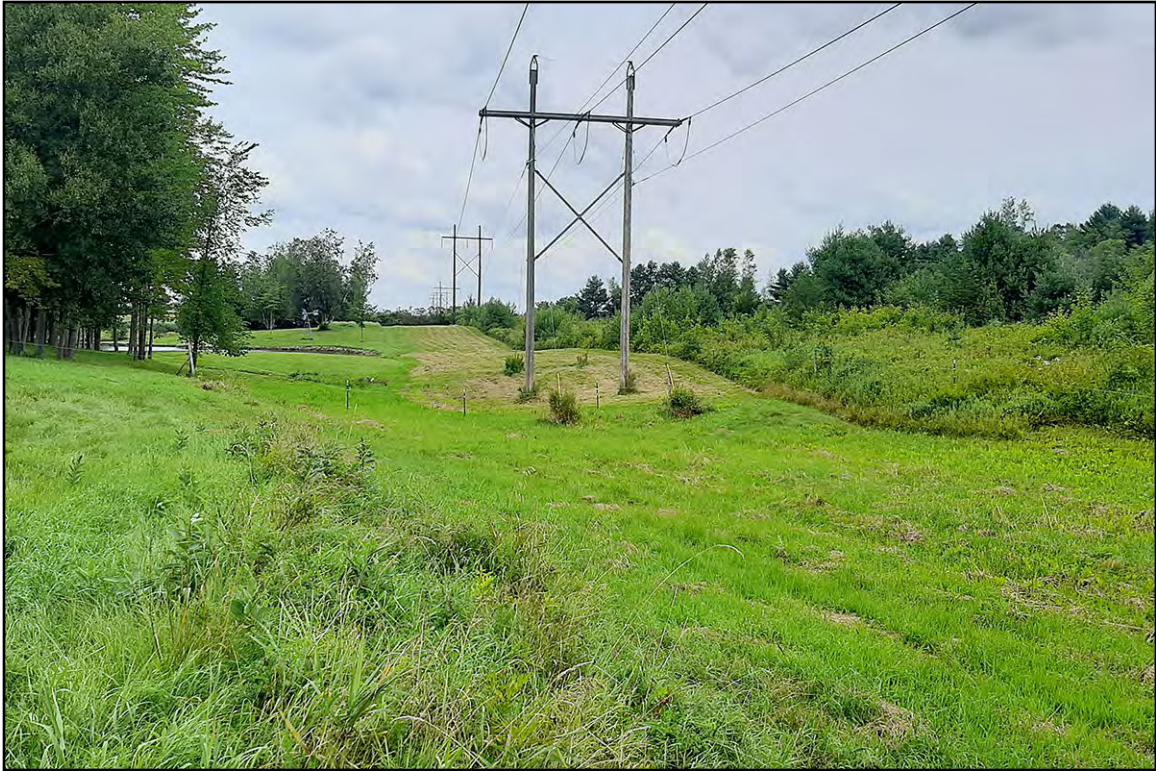
PLATE 155: Structure 219 with Pond and Standing Water, View North
