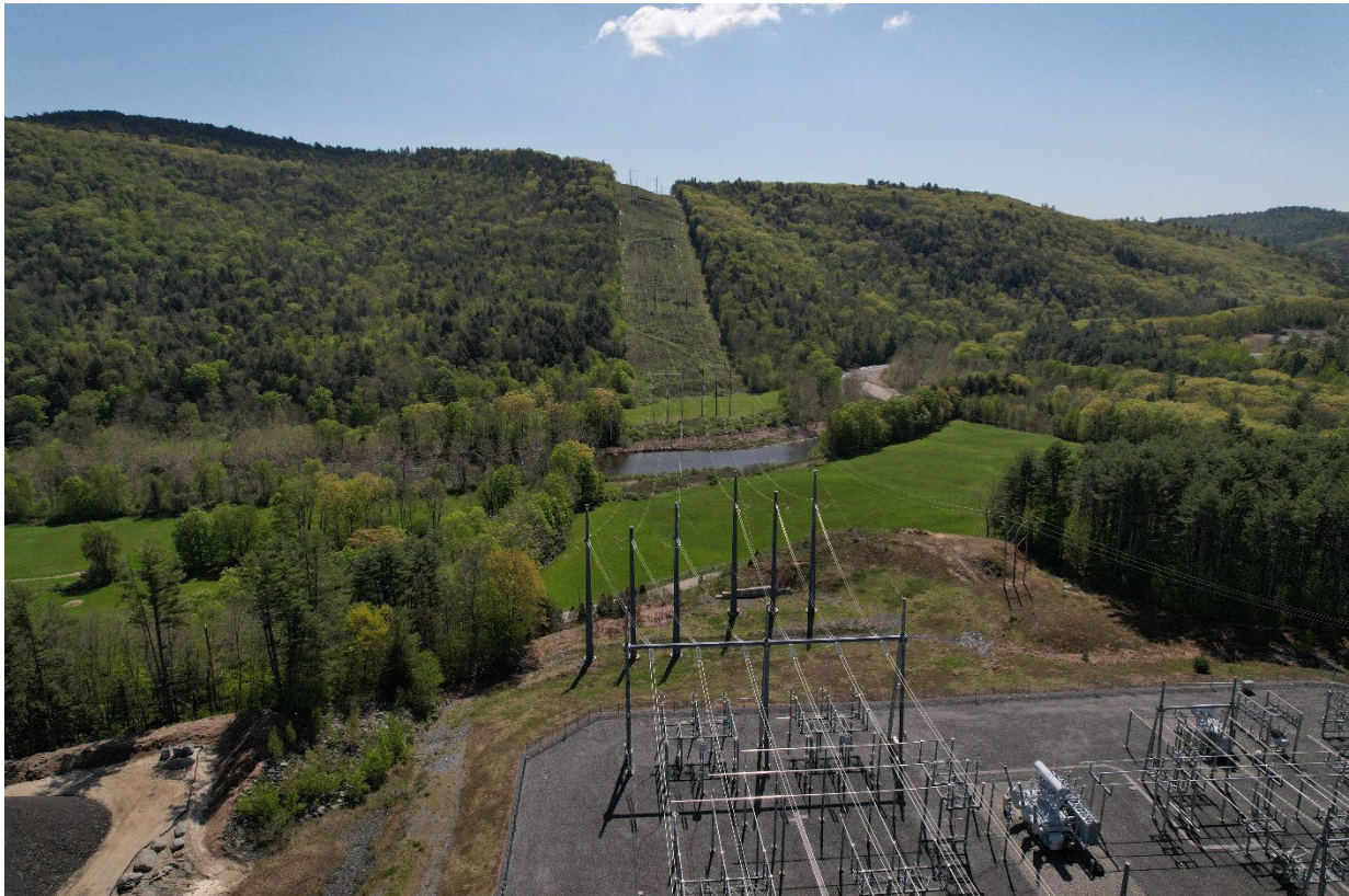
Photo by Jake Reed: Newfane Substation and Newfane Tap line
