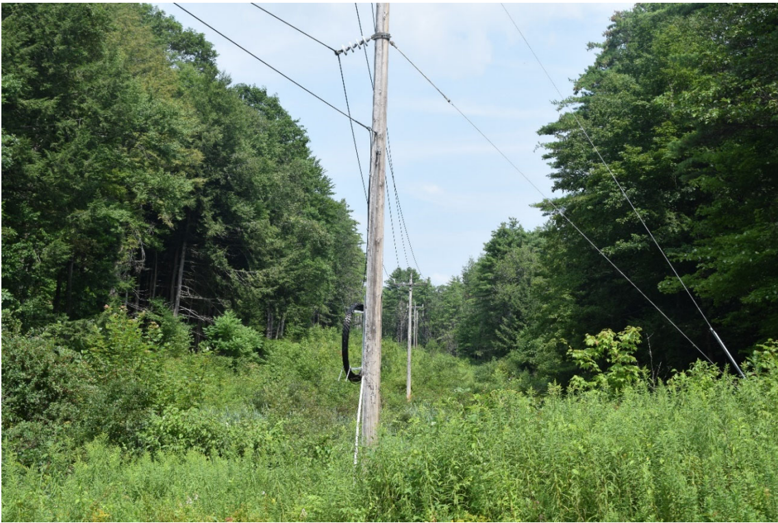
Photo 17. Project study corridor north of substation, view north; note visible slope from west to east.
