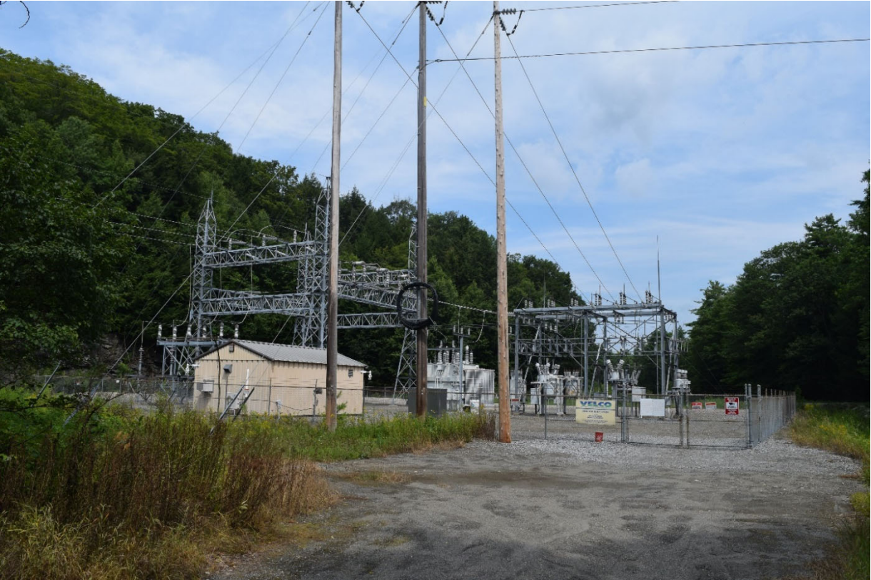
Photo 6. Windsor substation, view northwest.
