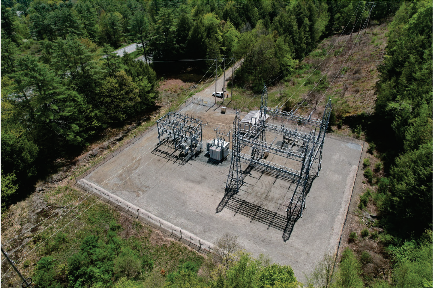
Figure 3: Oblique aerial view of the existing substation and surrounding overhead transmission and distribution facilities. This view is looking roughly south from the north, with I-91 visible in the upper left side of the image.
