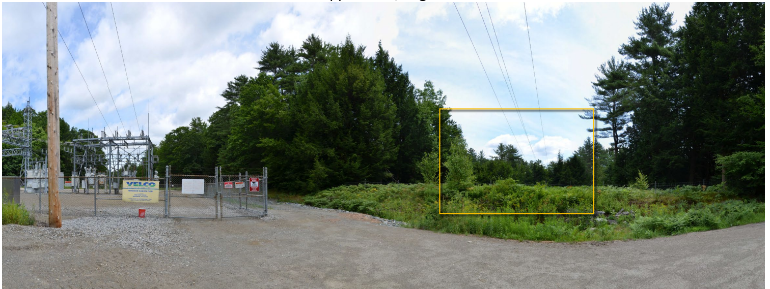
Viewpoint 1: Approximately 180° panoramic view from the existing substation access drive, West of Interstate 91, panning from roughly north (left) to south (right). The orange rectangle represents the image below, which is captured with a 50mm equivalent lens.
