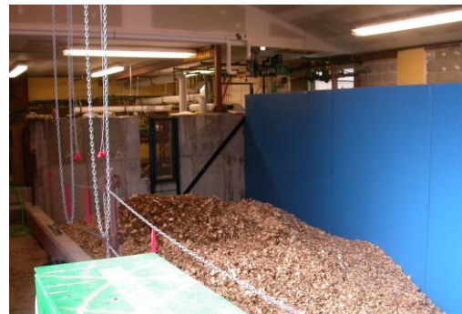
Figure 27: Wood chip heating system at Weathersfield School.
