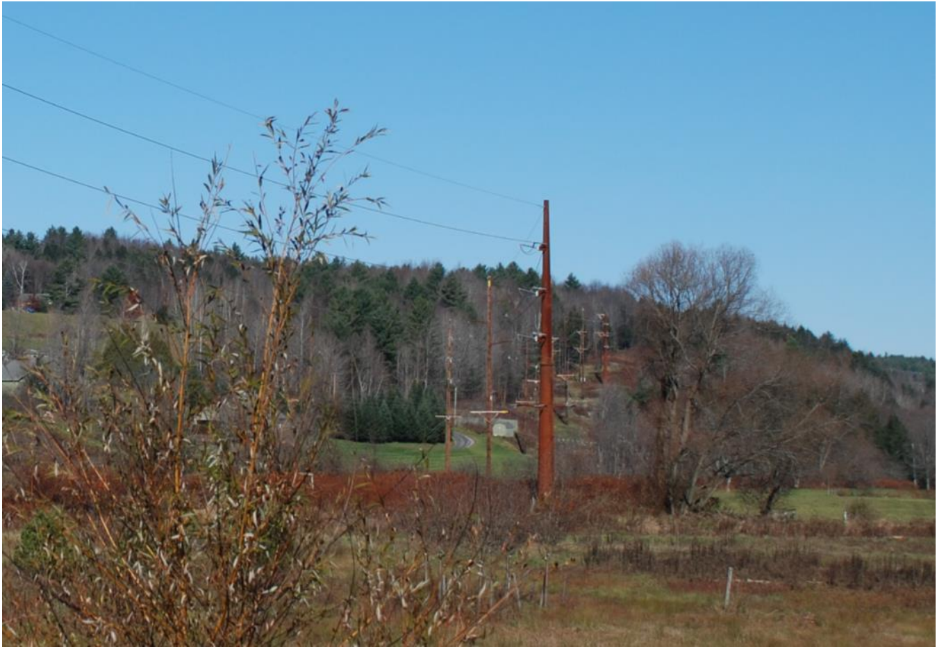
Figure 2: Image showing an existing self-weathering steel structure on the K24-5 line near Moscow Road in Stowe, VT.
