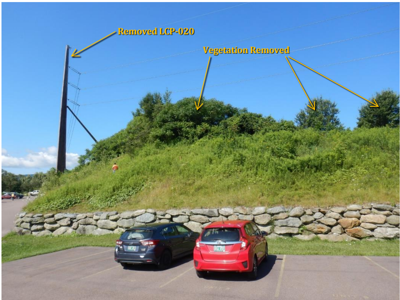
Figure 1: Image showing original laminate wood structure #LCP-020 prior to removal of the structure and some of the existing vegetation.
